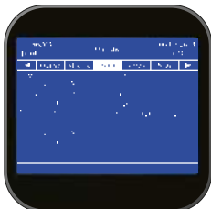
UPS Cabinet Control Panel
